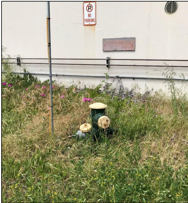
Reservoir Suction Hydrant
