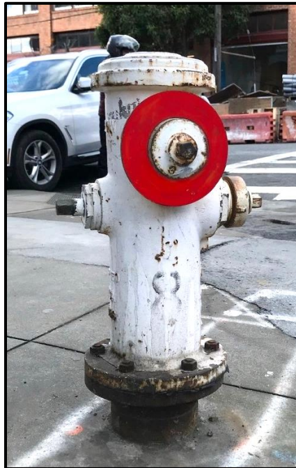
Out-Of-Service Low Pressure Hydrant
