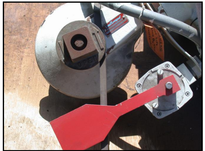
Motorized Valve in the Local (Manual) Position
